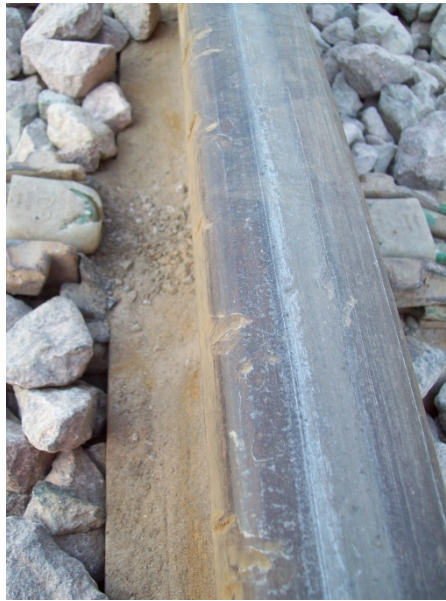
Figure 36 Damaged rail due to excavator impact (Image courtesy of Robert Langford)
