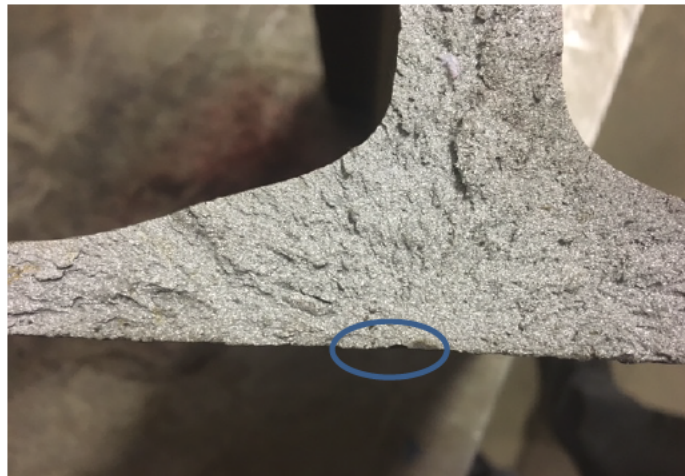
Figure 2 Broken Rail showing a corrosion pit
