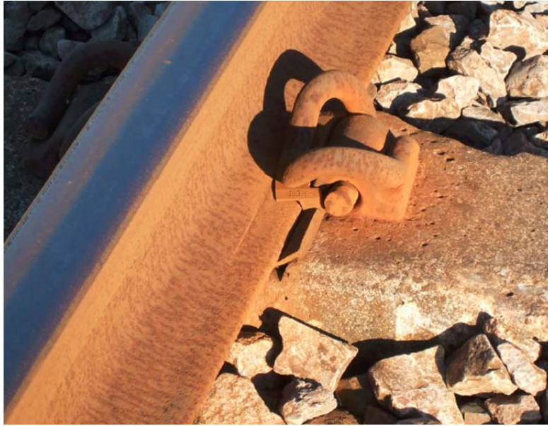
Figure 30 Wear to sleeper caused by attrition from worn rail seat pad (Coverdale & Jones, 2011)
