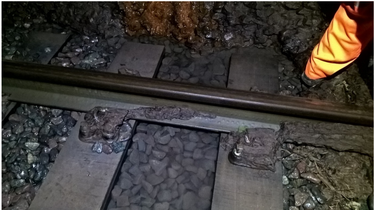
Figure 38 Example standing water causing track deterioration Kilsby Tunnel
