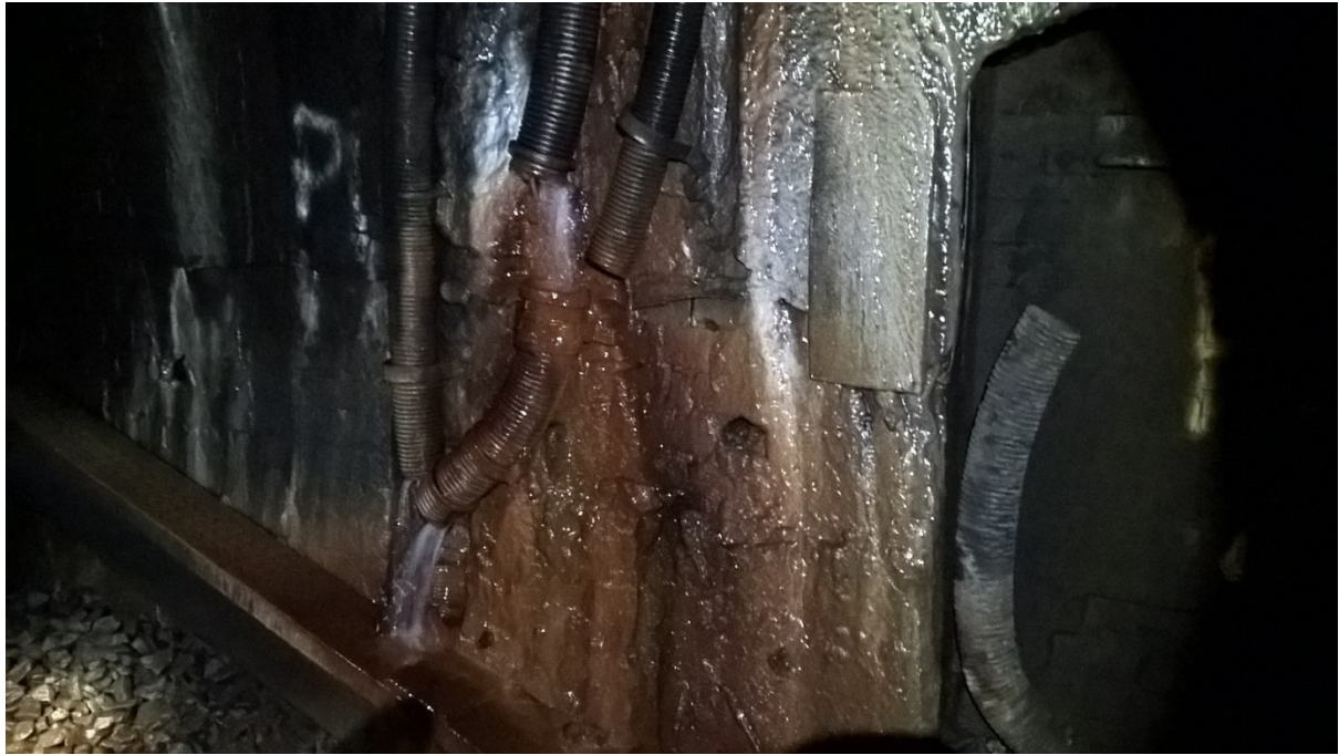
Figure 37 Example ineffective structure drain Kilsby Tunnel
