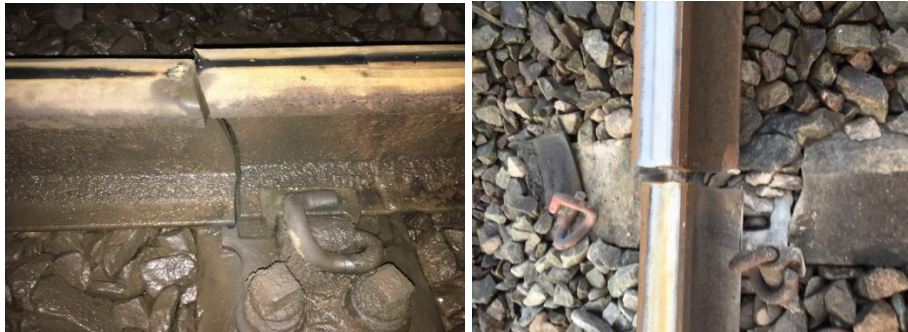
Figure 15 Photos from TEF3064 reports of actual broken rails from Kilsby Tunnel and Bourne End on the West Coast Main Line respectively
