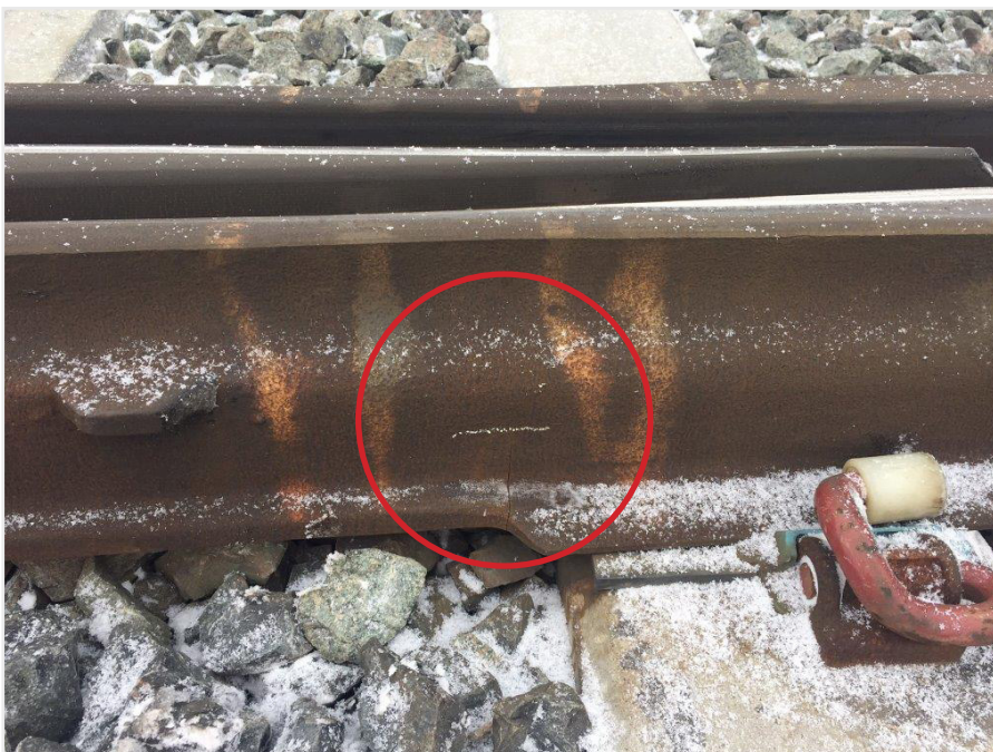
Image 1: Example of a fatigue crack on a crossing
