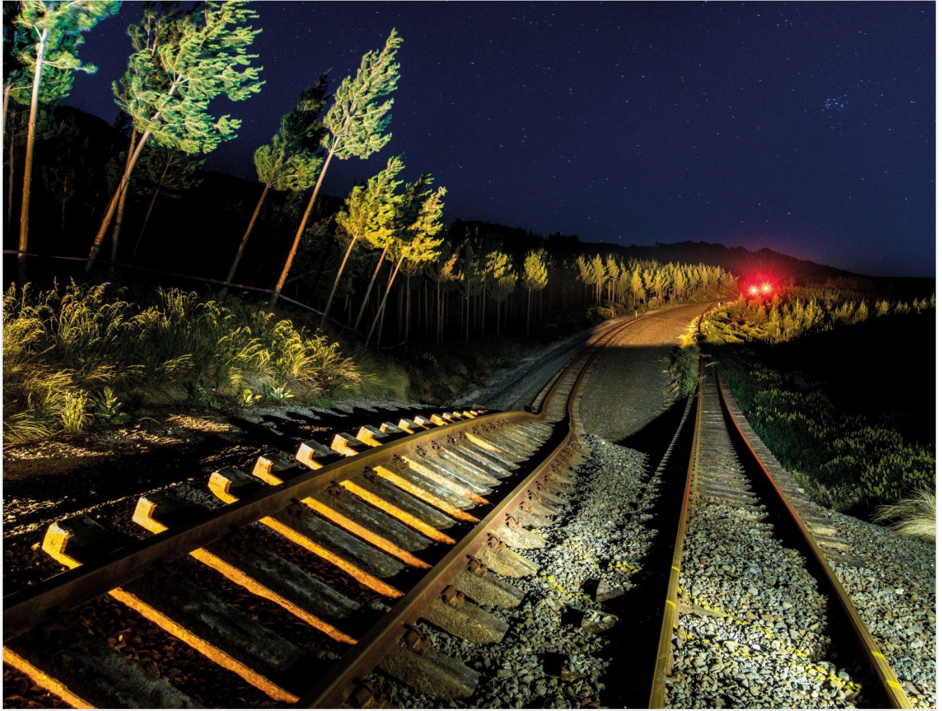
Image 5: A twisted and contorted permanent way north of Kaikoura. Photo courtesy of KiwiRail
