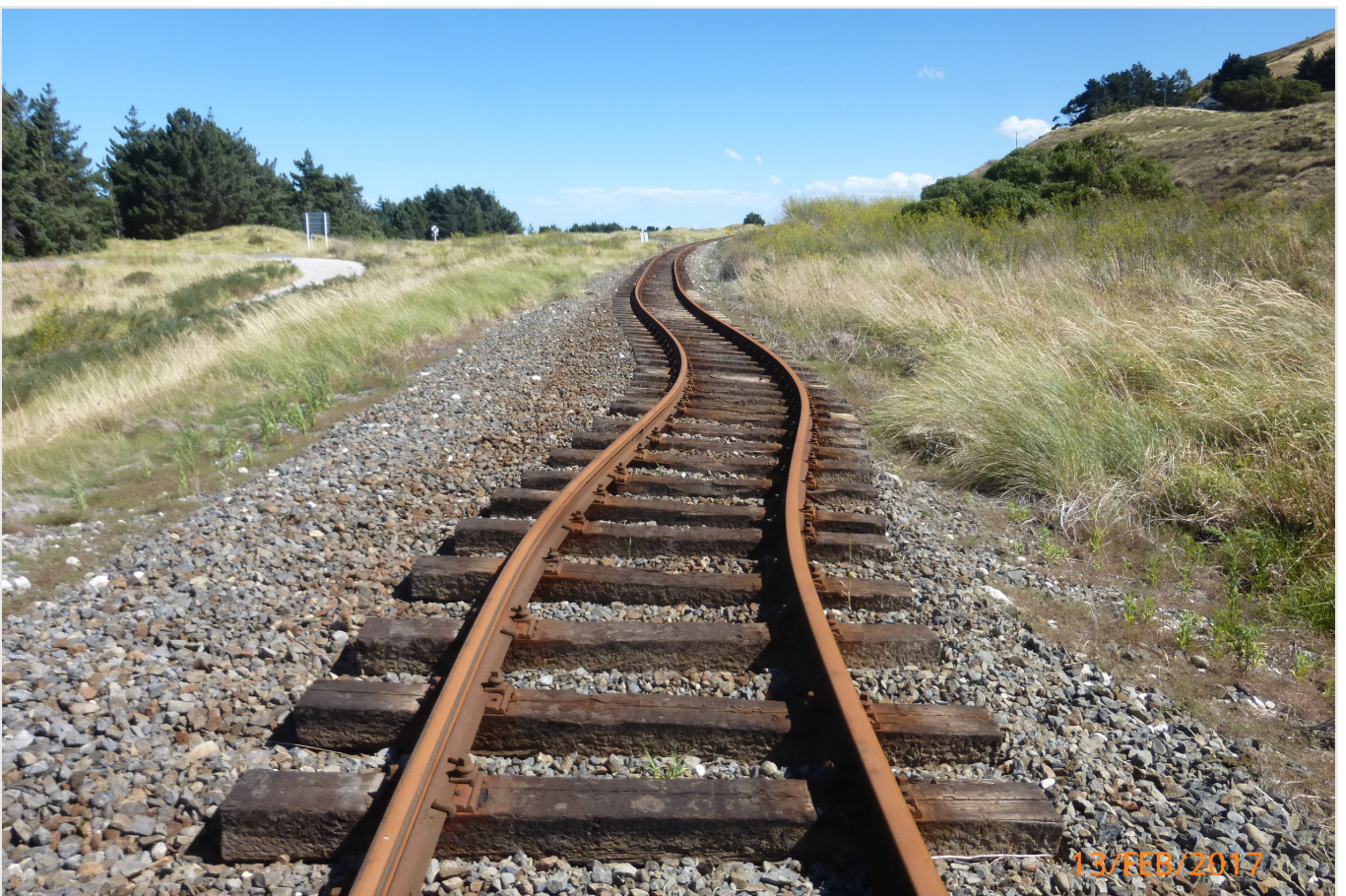
Image 7: Permanent Way damage south of Blenheim. Photo by Phil Kirkland
