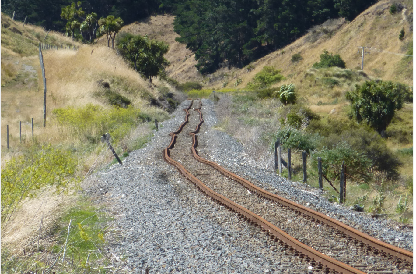
Image 6: Permanent Way damage south of Blenheim. Photo by Phil Kirkland
