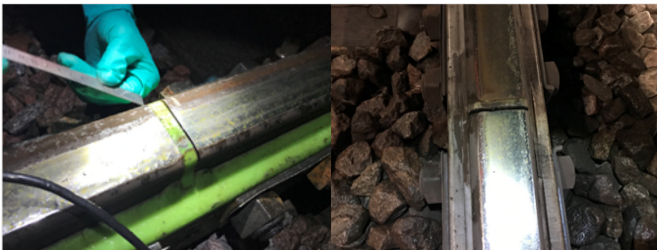
Figure 9: Endpost filler voiding
