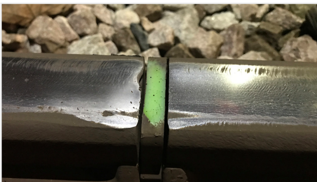
Insulated rail joint (IRJ)
