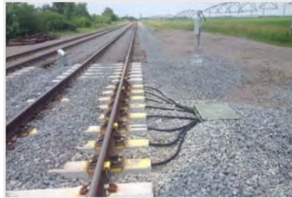
Figure 10: Wheel Impact Load Detectors; NS WILD using the Salient process installed on heavy tonnage mainline at Flat Rock, Kentucky in 2009 (top) and CSX WILD using the Schenck process on mainline at Webster, Indiana (bottom).
