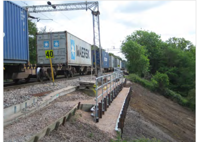
B) 50m 73 to 75ch Up. Two rows of cess retention constructed during May 2011, the slope continued to deteriorate shortly after construction due to deep seated failure (Ref 11)
