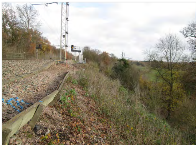
A) 49m 71ch Up. Exposed sleeper ends, ballast spilling down slope and failing cess
