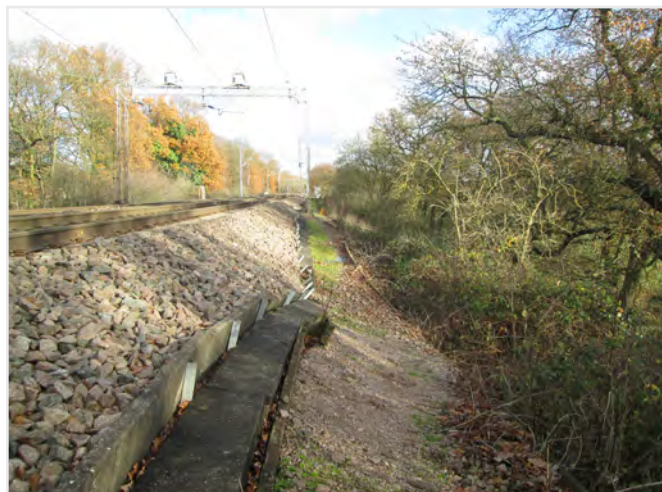
B) 49m 78ch Up. Large dip in cess walkway and associated track dip
