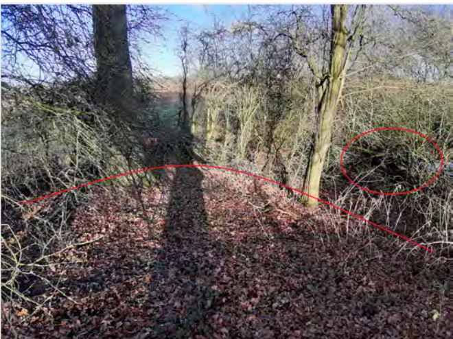
E) 49m 76ch Down. Historic toe bulge blocking toe ditch causing ponding at slope toe
