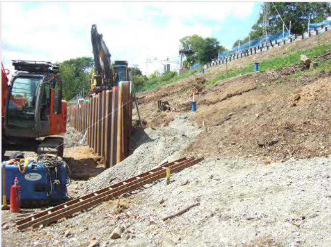
C) 50m 73 to 75ch Up. Sheet pile wall constructed in summer 2011 to replace the failing cess retention and address deep seated failure mechanism (Ref 12)
