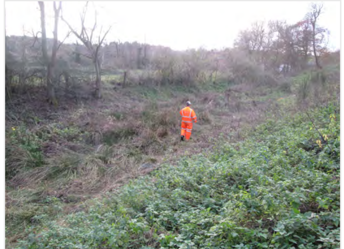
B) 49m 74ch Up. Hydrophilic vegetation and ponding at toe beneath sheet pile wall earthwork renewal
