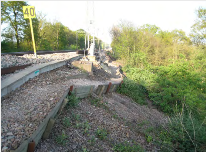
A) 50m 73 to 75ch Up. Distorted cess walkway and temporary speed restriction (TSR) speed board, in early 2011 prior to remediation
