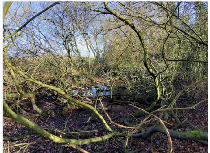
D) 49m 77 to 78ch Down. Ponding at slope toe – opposite worst defect on Up Side
