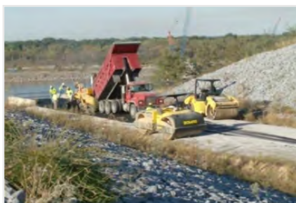
Fig 8 Bridge approaches; Portion of the 425 m, (1400 ft), CSX Tennessee River bridge approaches placed in 1998; note the paved shoulders between wingwalls to intercept water (top) and similar project on Paducah & Louisville Railroad showing asphalt paving for the east approach to the new bridge across the Tennessee River in far West Kentucky (bottom). The bridge approaches have required minimal maintenance.
