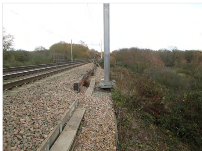
D) 50m 15ch Up. Sleeper ends exposed, poor cess condition. A small king post retaining wall has been constructed to retain ballast at this location.
