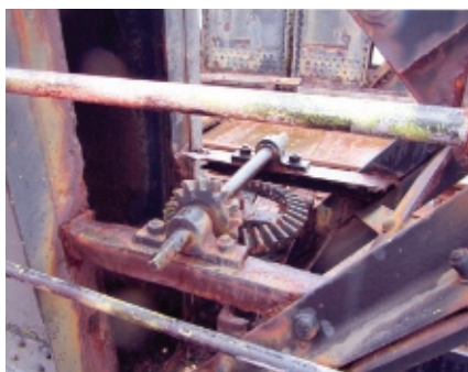
Some of the former hand-operated swing bridge section rotational gear. The seaborne wind, salt air and wetness are reflected by the state of rusted members. Tubular walkway handrails run along the bowstring sections (photo by Robert Hyett).
