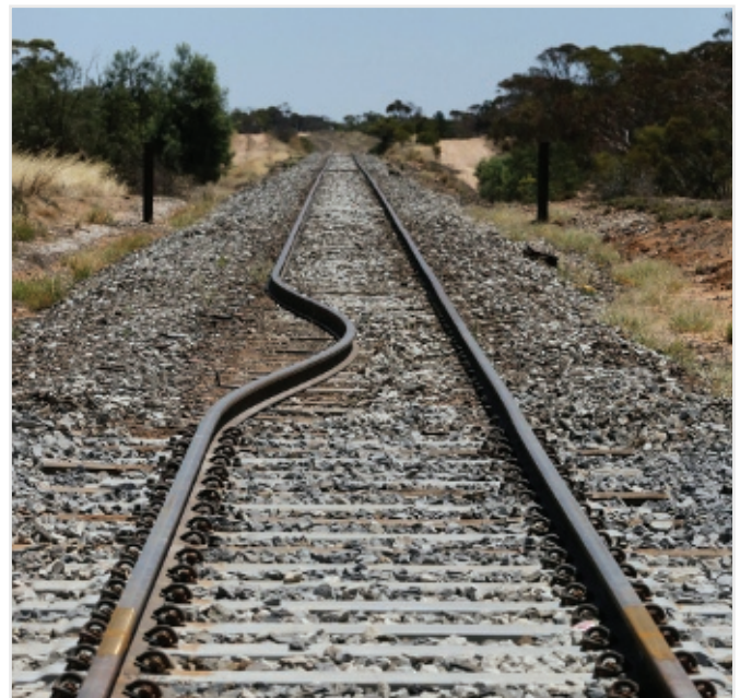
Image 6: The impact of thermal stresses in CWR. Here the weak point in the new works appears to be where the new concrete sleepered track adjoins existing timber / spiked track. Thermal stresses have overcome the weaker track fixings (image: WCC).
