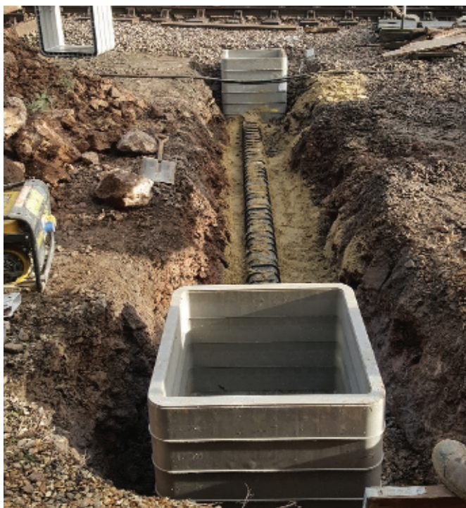
Image 4: Installed UTX prior to filling in.
