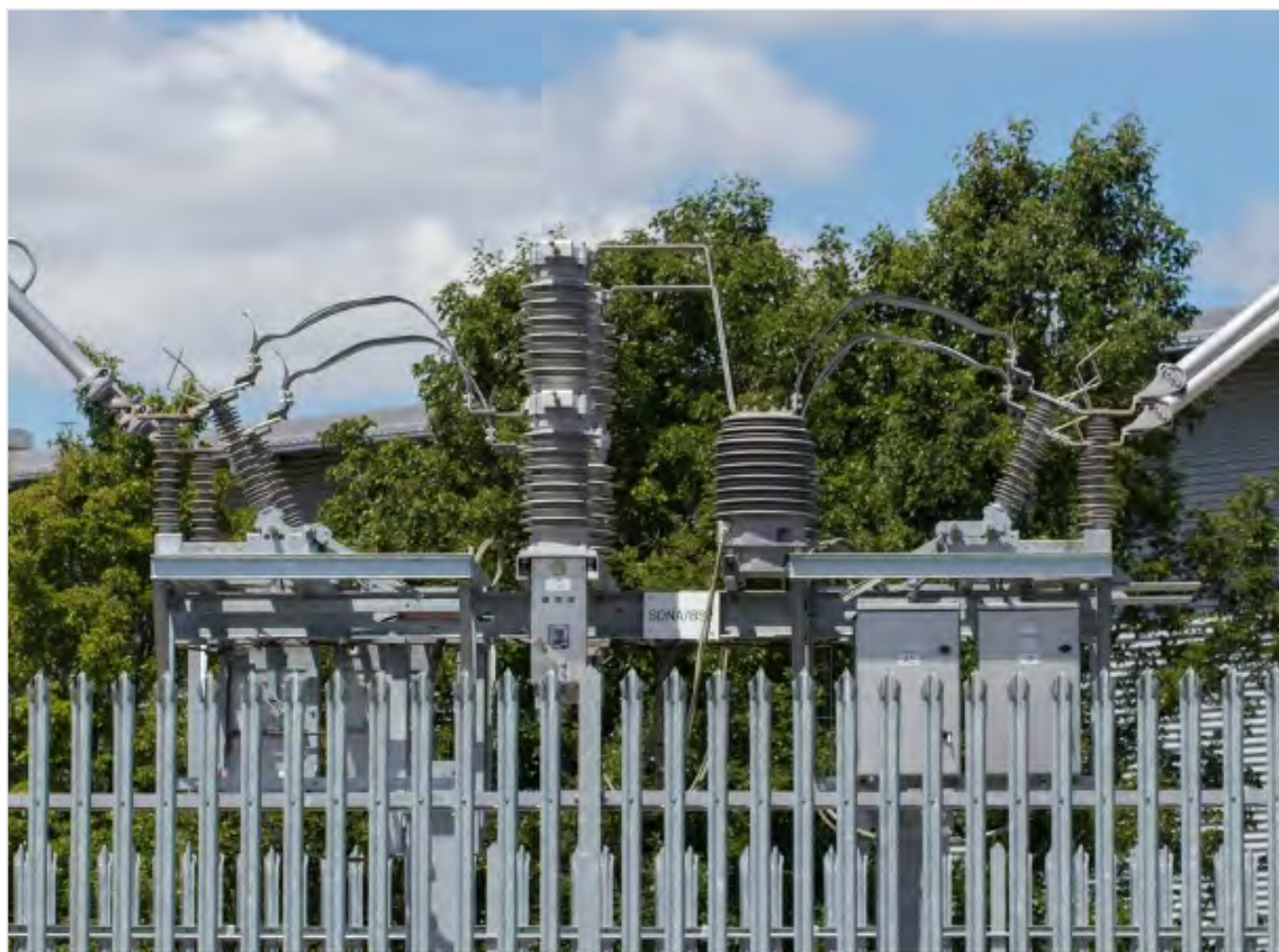
Figure 2: SF6 circuit breakers (photograph: Garry Keenor).
