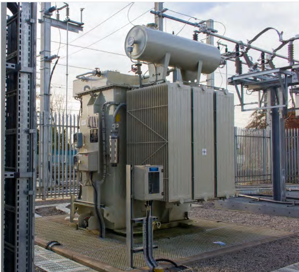
Figure 1: An autotransformer within a traction substation compound (photograph: Garry Keenor).
