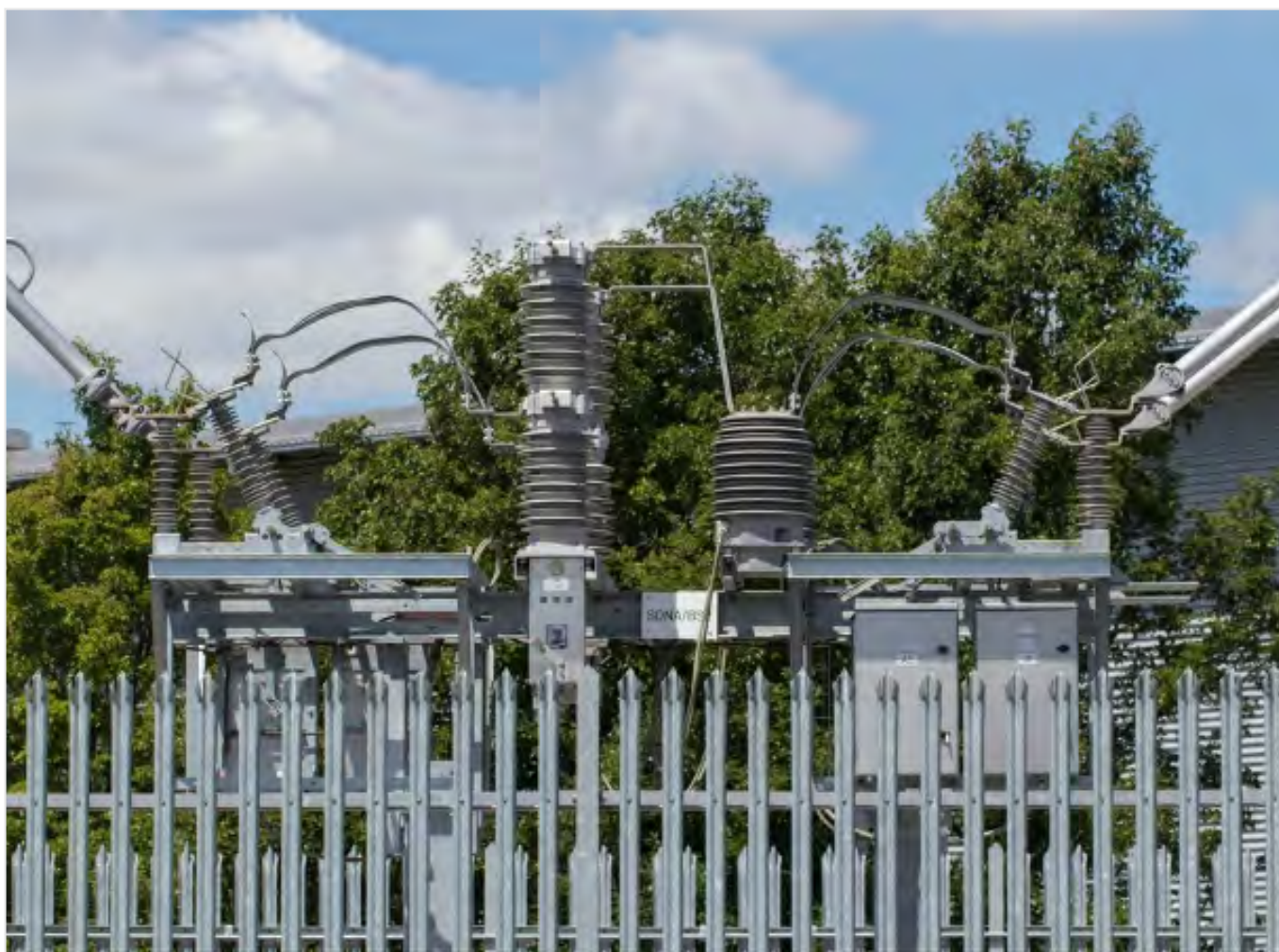
Figure 2: SF6 circuit breakers (photograph: Garry Keenor).
