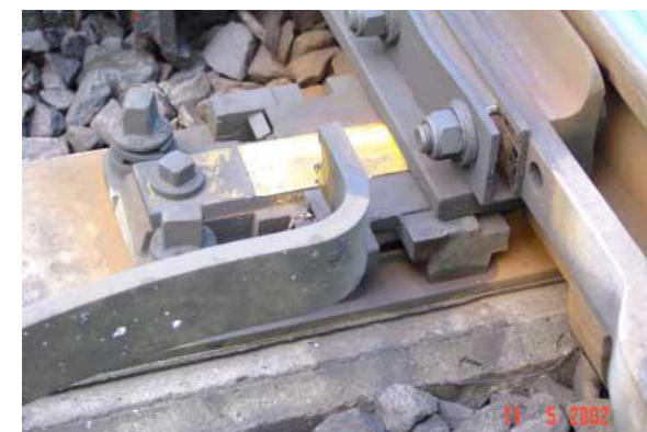
Photo courtesy of: Potters Bar fractured lock stretcher - HSE
