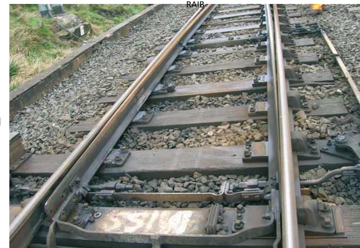
Photo courtesy of: Grayrigg defective switches - RAIB
