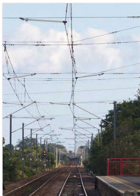
Figure 8: Contact wire stagger (zigzag) on tangent track; East Boldon, UK
