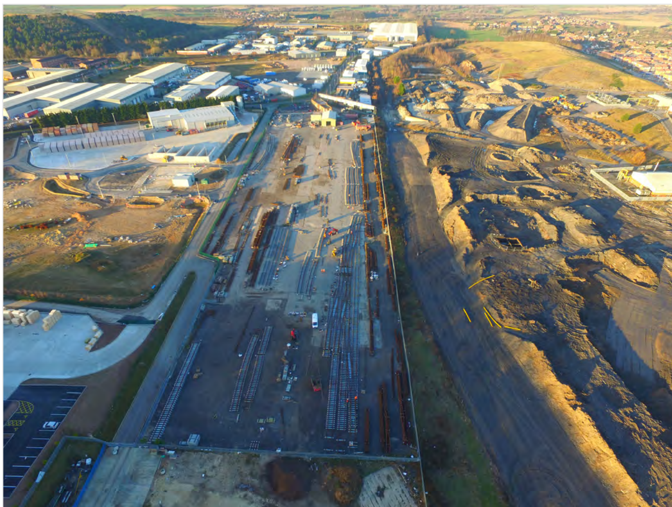
Figure 7: S&C assembly needs space! VAE's 18,000 square metre layout ground at Harworth near Doncaster
