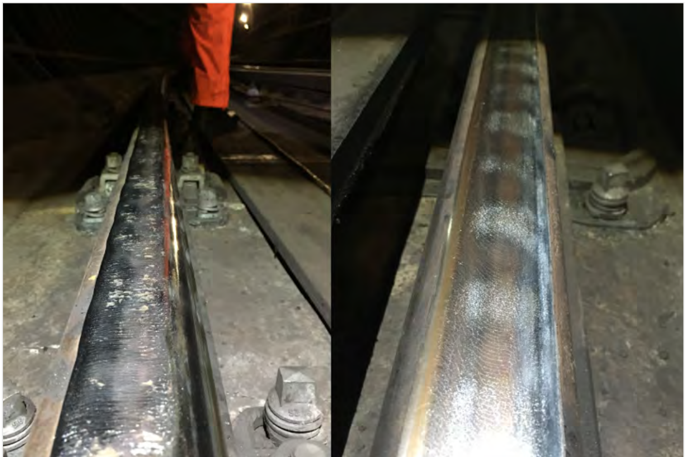
Figure 13: Rutting corrugation on modern track-form
