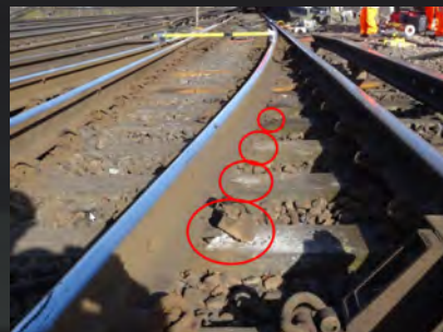
Image 4: Eastleigh derailment 28 January 2020 - The broken fastenings
