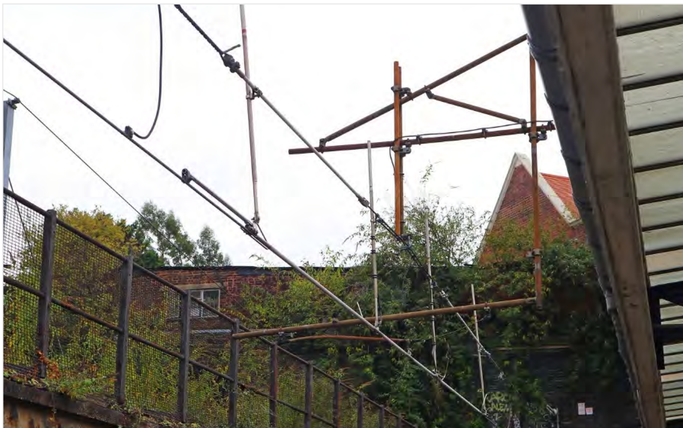
Figure 17: Arthur Flury type inline neutral section; Drayton Park, UK. Note the uninsulated cantilever at the neutral point
