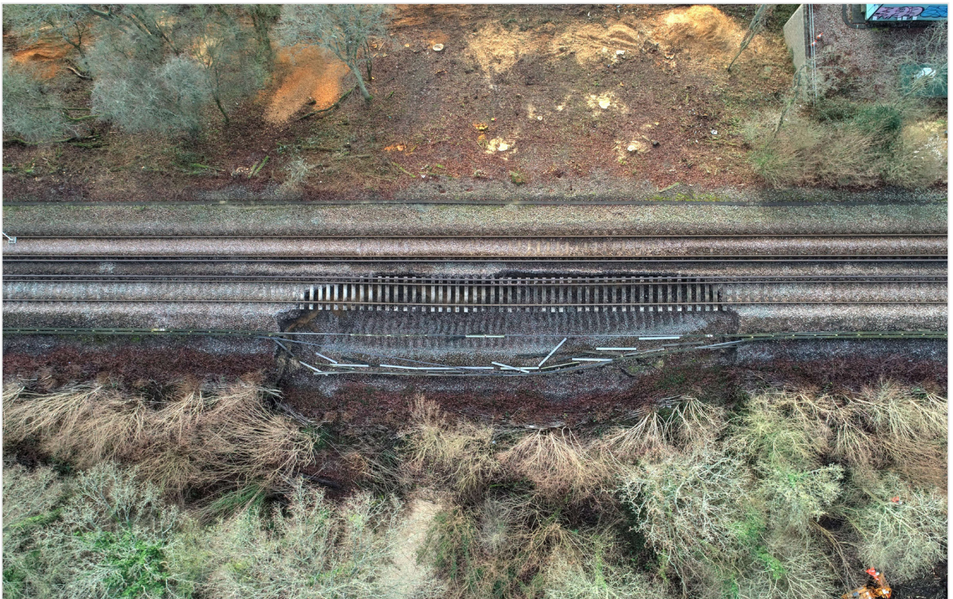
Figure 5: Drone footage of failure site from 2019/20.
