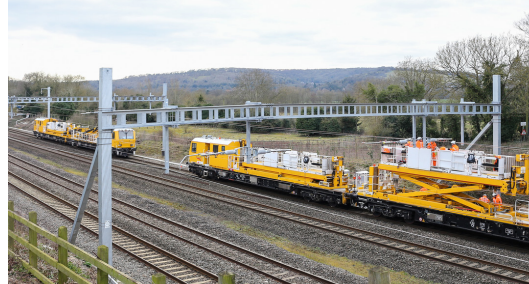
Network Rail Factory Train
