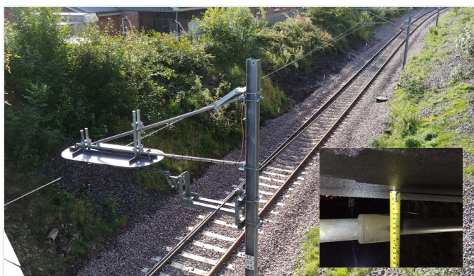
Figure 12: Voltage-controlled clearances trial installation – Paisley canal (Scotland's railway).
