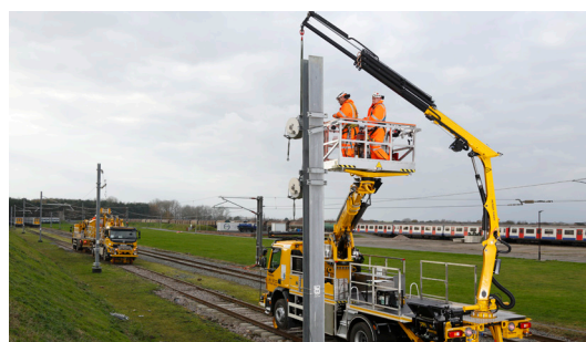
Mobile Elevating Work Platform (MEWP) unit developed recently for electrification work
