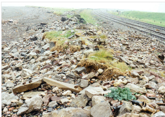
Figure 15: Exposed location at Siddick showing continual erosion.
