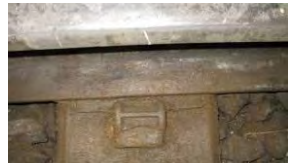
Above: rapid rail corrosion in new rail installed only 3 months earlier
