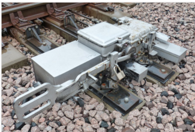
Figure 1: A point machine with integral levers for manual operation and for switching between auto and manual (Photo Francis How).
