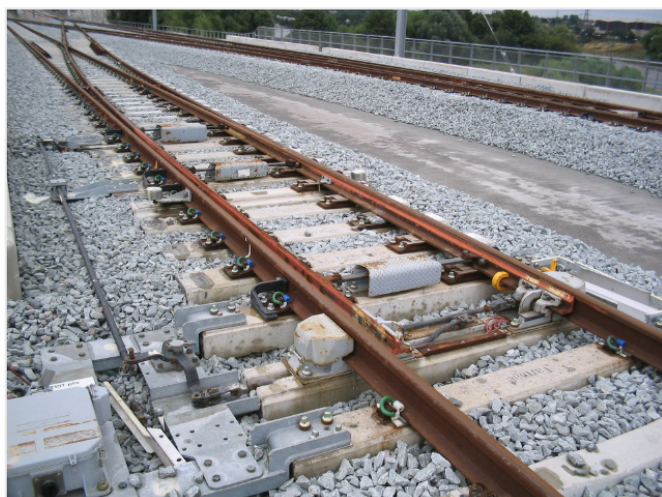
Figure 2: A set of points fitted with a back-drive on the left-hand side. The bracket connected to the sleeper at the intermediate stretcher bar position supports the rodding run by way of a rodding roller wheel (Photo John Alexander).
