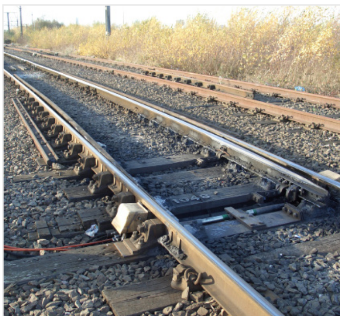
Figure 11: An example of a catch point that derails trains. Photo Network Rail.
