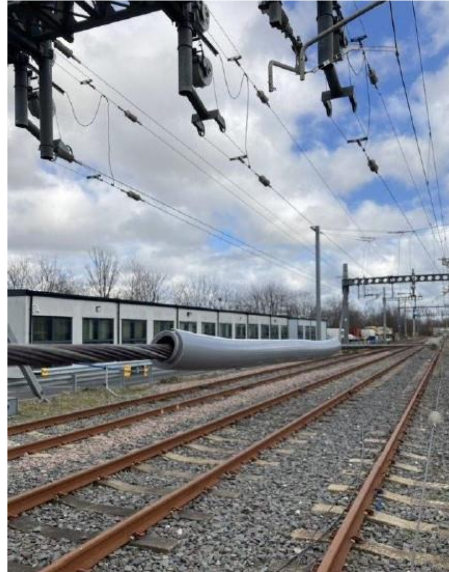
Line hose – secondary insulation
