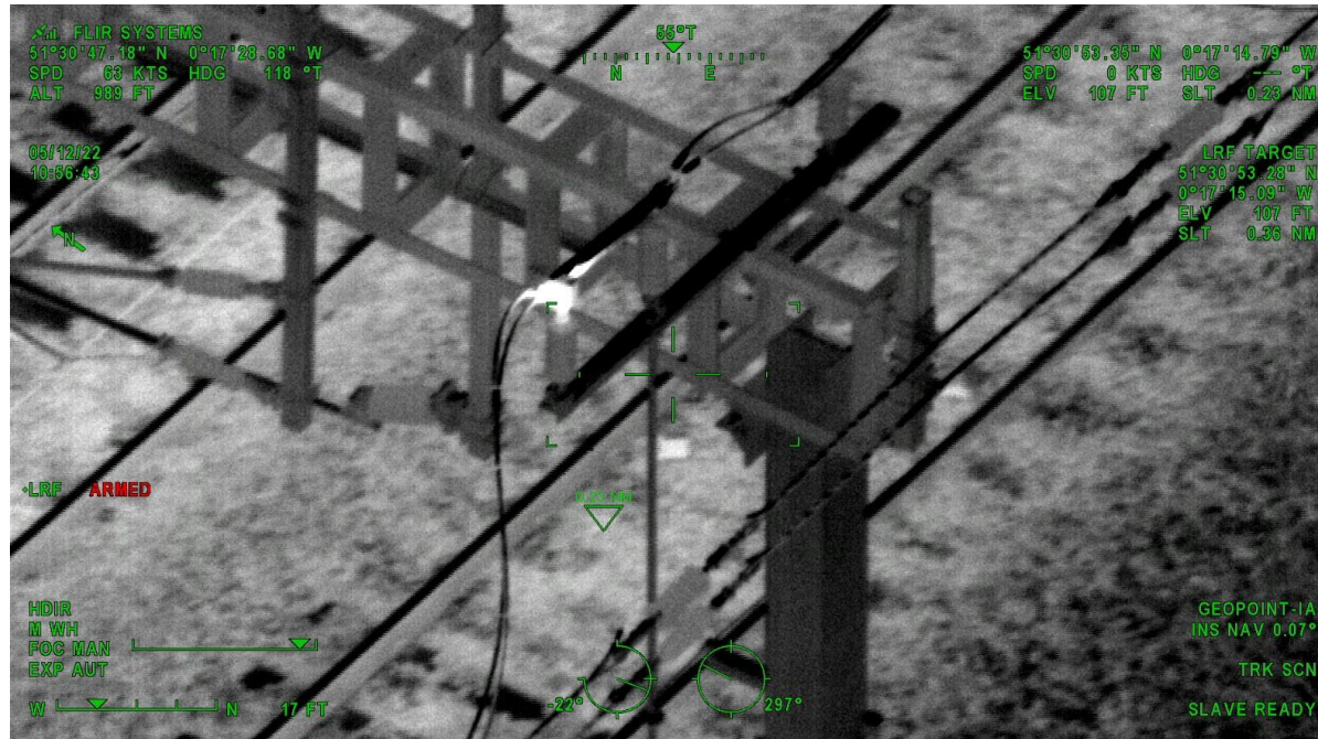
Thermal image of an isolator taken from a helicopter
