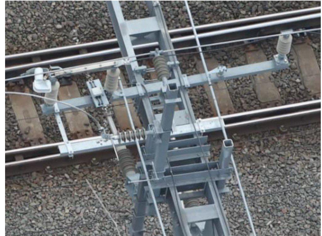
Image of an isolator taken from a helicopter
