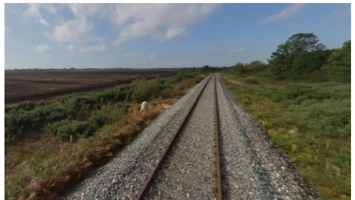
Figure 9: Site condition at Case Study 2, before Trackbed stabilisation
