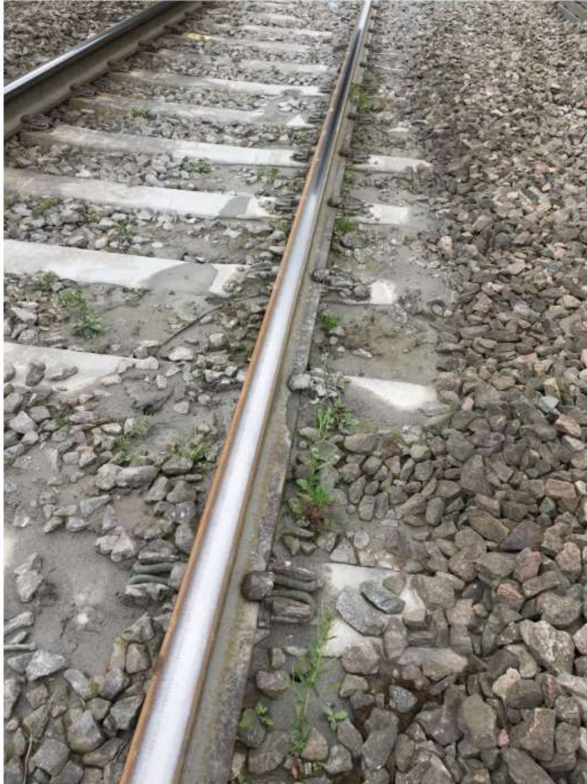
Silt, weeds and fines settled on the 6ft rail of the Down Charfield
