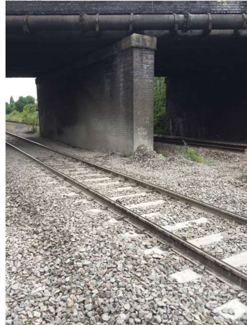
Visible slack under Stroud Road O/B, note excessive wet bed spoil around the area
