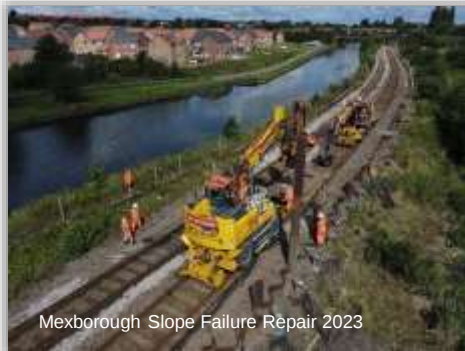
SPC1 Harlington Embankment Failure 2021
