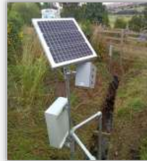
Remote Drainage Condition Monitoring Installation
