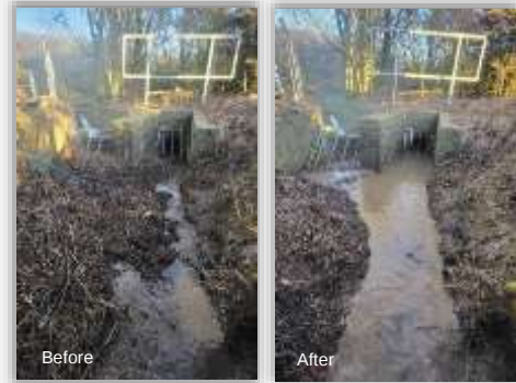
ECM1 Stoke Jn – Trash Screen Clearance Before/After
