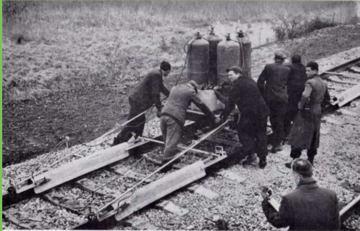
Rail heater at Bridgewater. (C. 36910)
