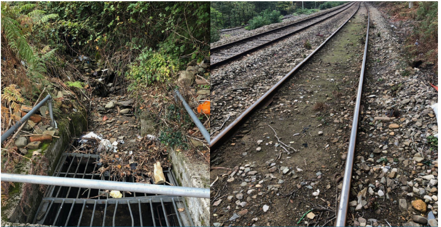
Figure 8: Adverse weather debris flow blocking flume to culvert, resulting in overtopping of headwall causing silt contamination of ballast and line closure
