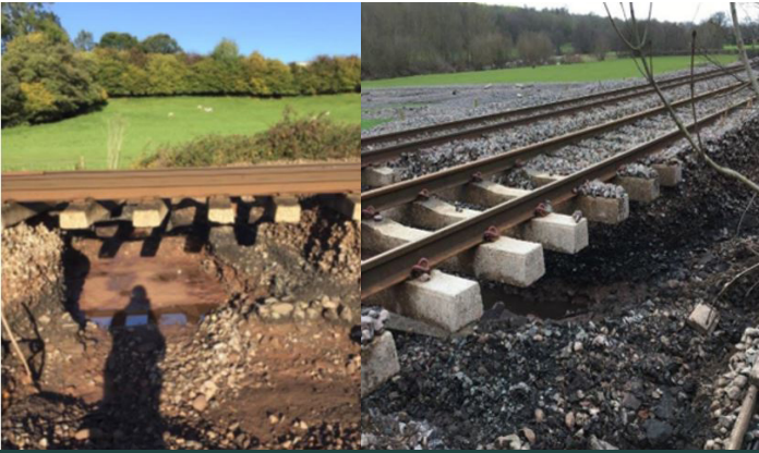
Figure 2: Images showing the damage from two different washouts in Winter 2019/2020. These washouts happened within 4 months of each other.
