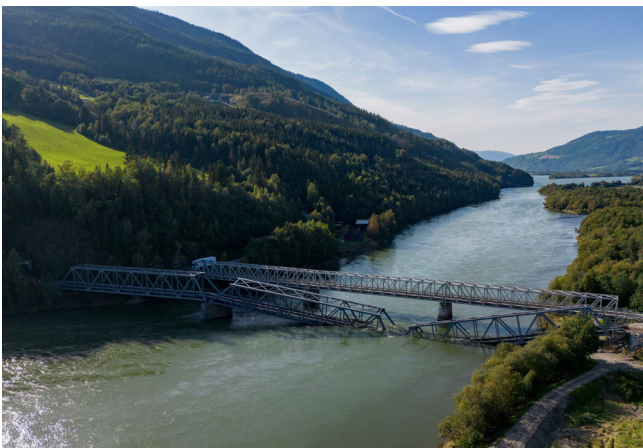
Figure 7: Norwegian bridge collapse.
