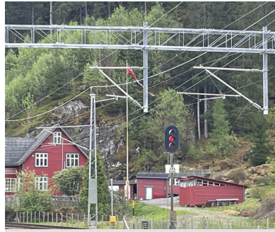
Figure 5: Modern Norwegian steel masts.
