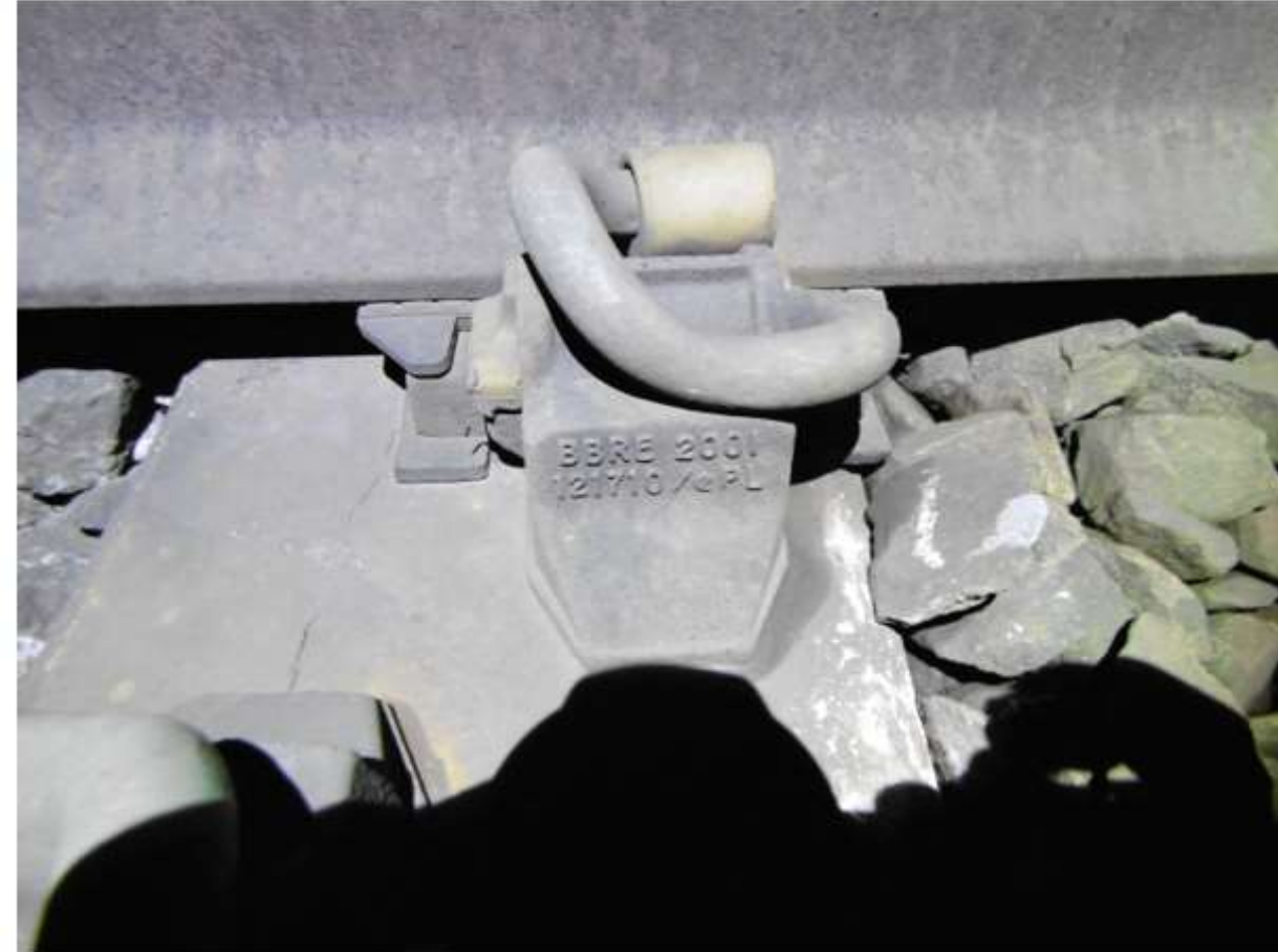
BH22A/B Pts – Typical cracks in bearers around housings
