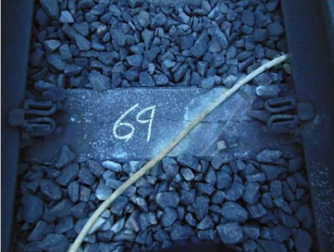
BH 48 Pts – Typical cracking in bearers
