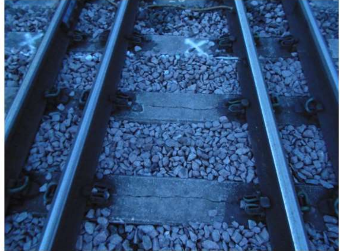
BH48/49 Pts – Typical cracking in bearers
