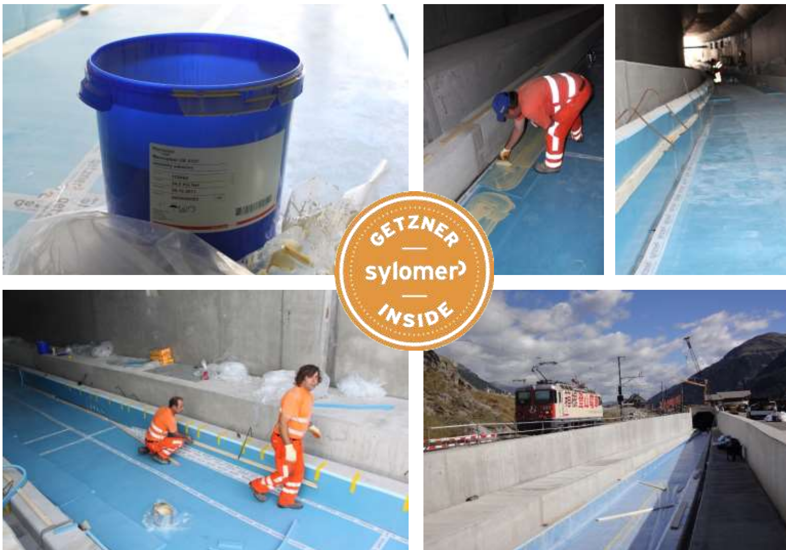
Project: Samedan, Switzerland
