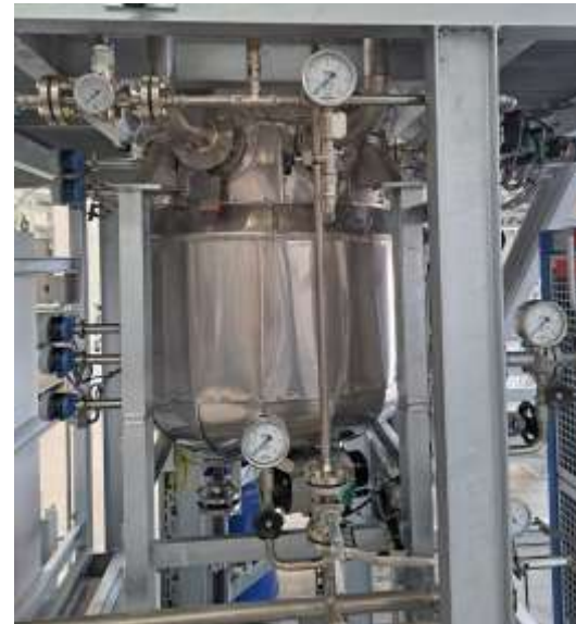
Recycled raw materials
