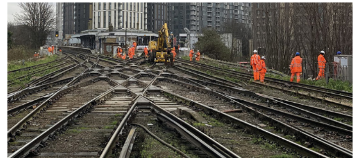
Figure 4: The former life expired Lewisham Junction showing signs of formation and Horizontal & Vertical alignment failure (Image courtesy of AECOM Form A).
