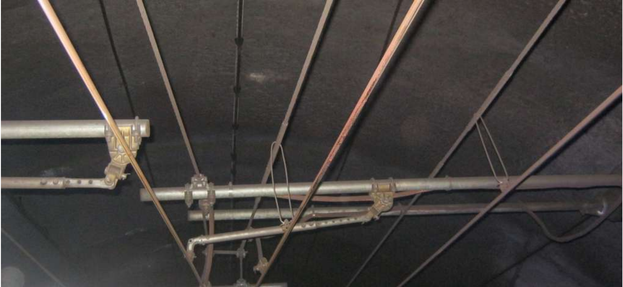
Example of the OLE inside Heathrow tunnels
