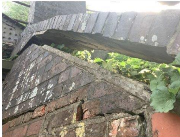
Photo No 11 - Low Mileage Downside Wingwall - Displacement - 0m From Downside - 22/09/2022
