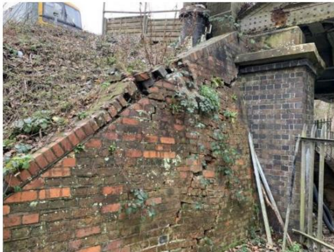
Photo No 18 - photo 18 low mileage upside wingwall - 27/01/2023
