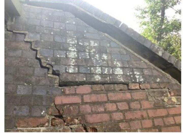
Photo No 10 - Low Mileage Downside Wingwall - Diagonal Fracture - 0m From Downside - 22/09/2022
