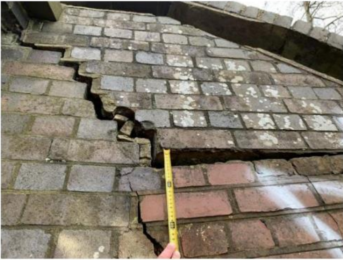
Photo No 17 - photo 17 horizontal fracture - 27/01/2023
