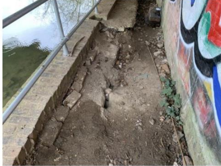
Photo No 25 - photo 25 void below abutment - 27/01/2023
