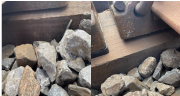
Figure 10: Chair lifting is present with AS screwspikes, and it was noted cracks appearing around holes which are failing to maintain a hold on the AS screwspikes.
