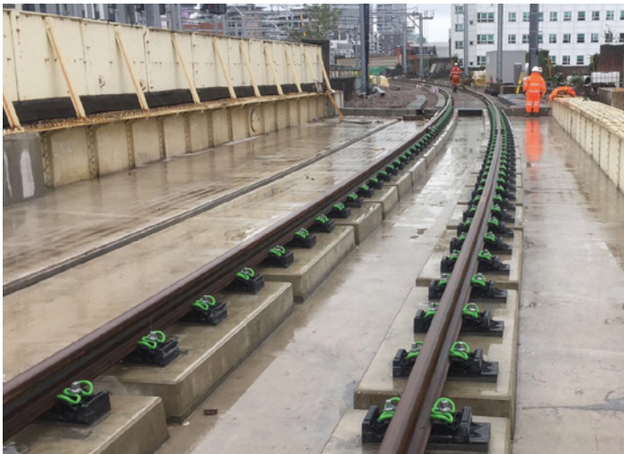
Figure 6: Longitudinal version of the IVES system as installed on viaduct at New Bailey Street, Manchester.
