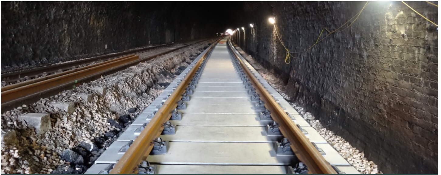
Figure 5: Standard version of the IVES system as installed in Asfordby tunnel in 2014.
