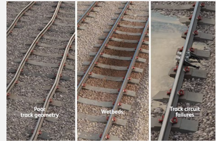
Image showing impact on track geometry from poor drainage
