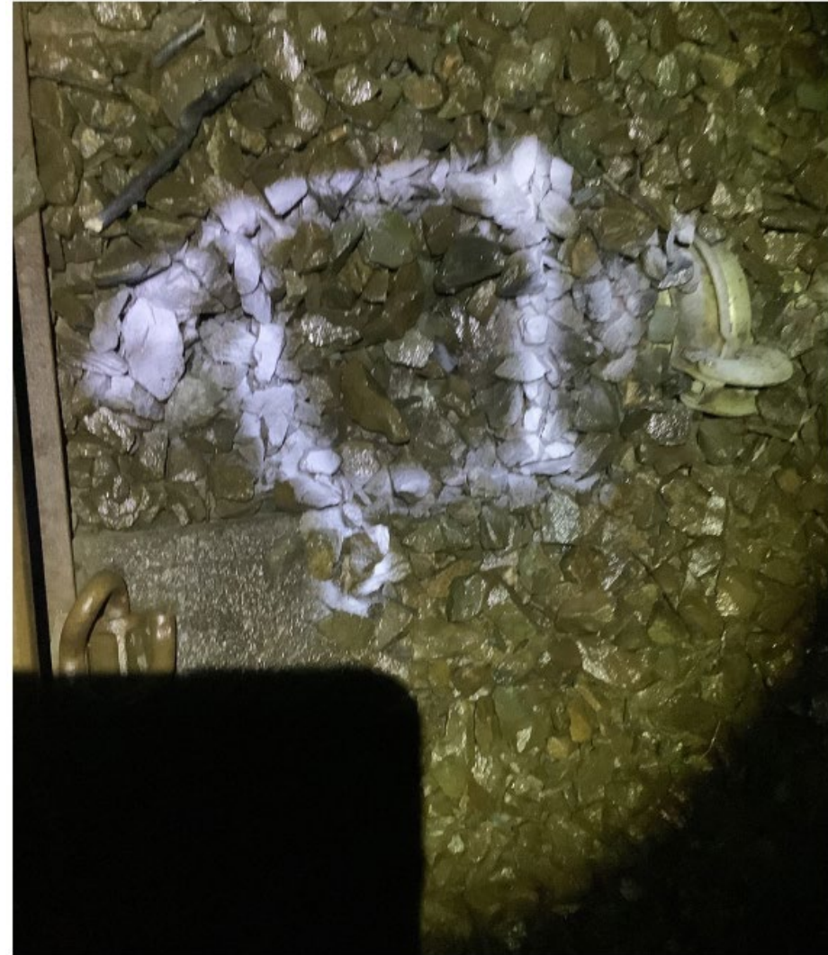
Damage to Pipe (Image: Network Rail)
