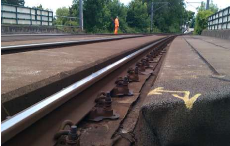
Existing PAN9 installation
