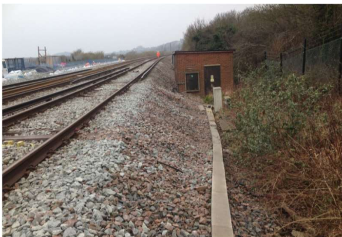
Folkestone Warren – Ballast Loss & Damaged Cable Trough
