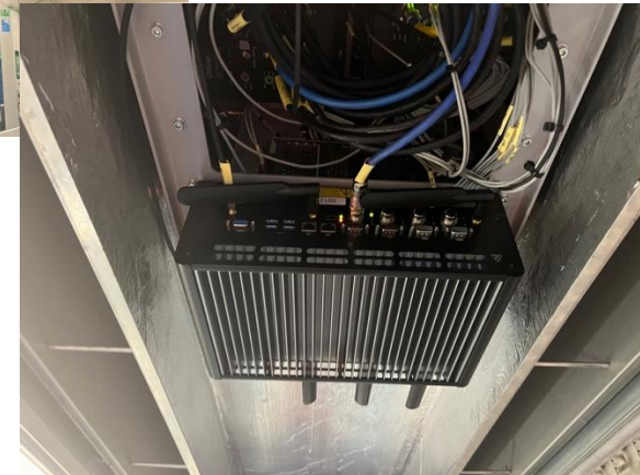
Processor installed in roof cavity of the train
