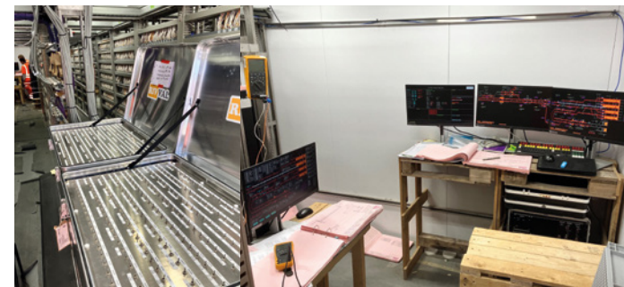
Figure 2: Grand Central Interlocking Test Westcad and Test Desks (Photo courtesy of the Authors).
