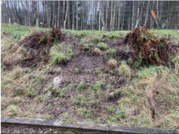
Figure 10: example of shallow failure on the HGL2 at approximately 8 miles 0670 yards, facing the Down side cutting face.
