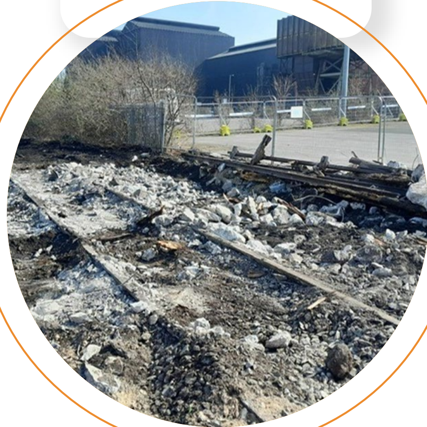
Contaminated material in the redundant steelworks siding to be removed
