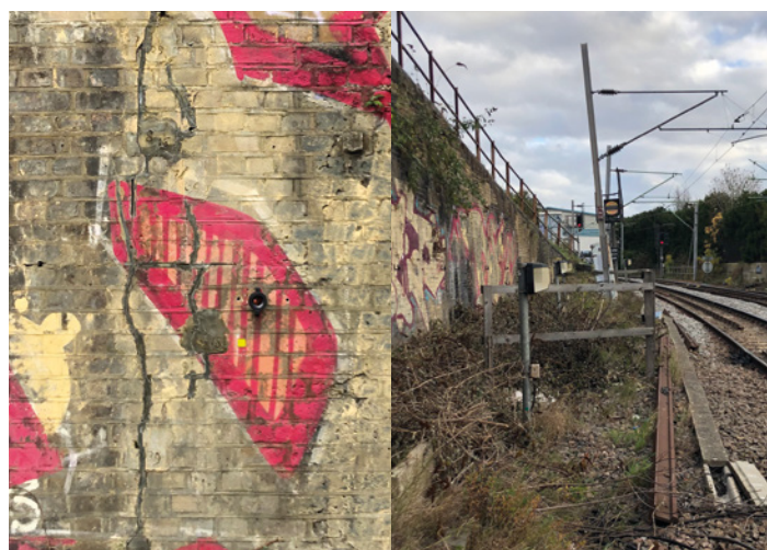
Figure 2: Evidence of deep-seated movement at the embankment toe, including distortion of OLE and signalling assets and historic repairs to the bridge wingwall.
